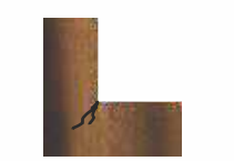
NO CLAIM WILL BE ENTERTAINED FOR CRACKING ARISING FROM GROOVE OR L-SHAPE CUTTING
